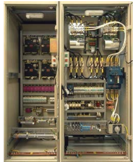
Part of a PRISMIC® A50 excitation system for a 259MVA turbogenerator
