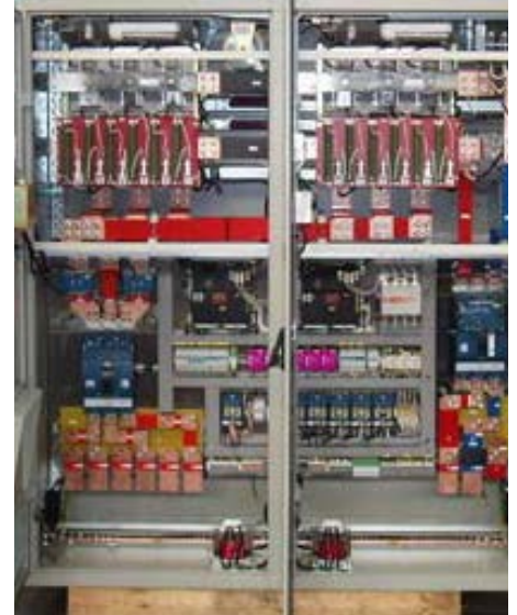
A BRUSH excitation system utilising modular power converters for a 140MVA turbogenerator
